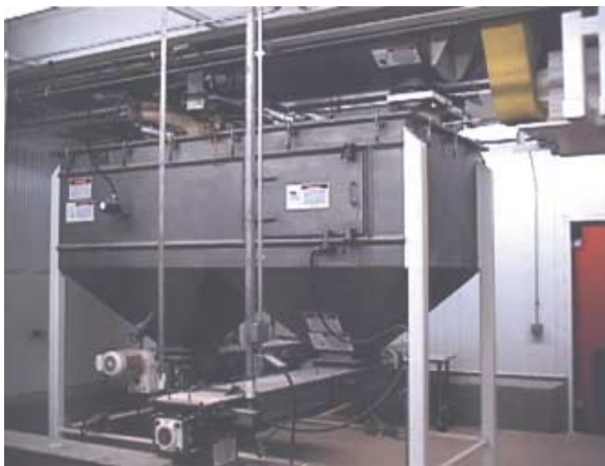
Three discharge valves in the blender's bottom allow for rapid material discharge to the surge bin.
